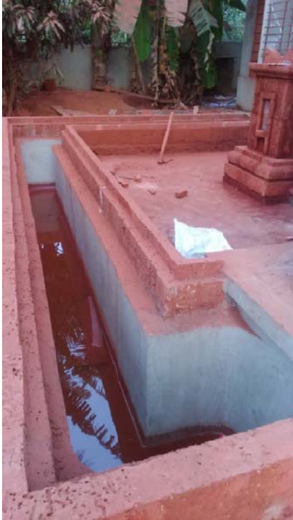
Figure 10: Water Harvesting Tank below the raised seating in courtyard
